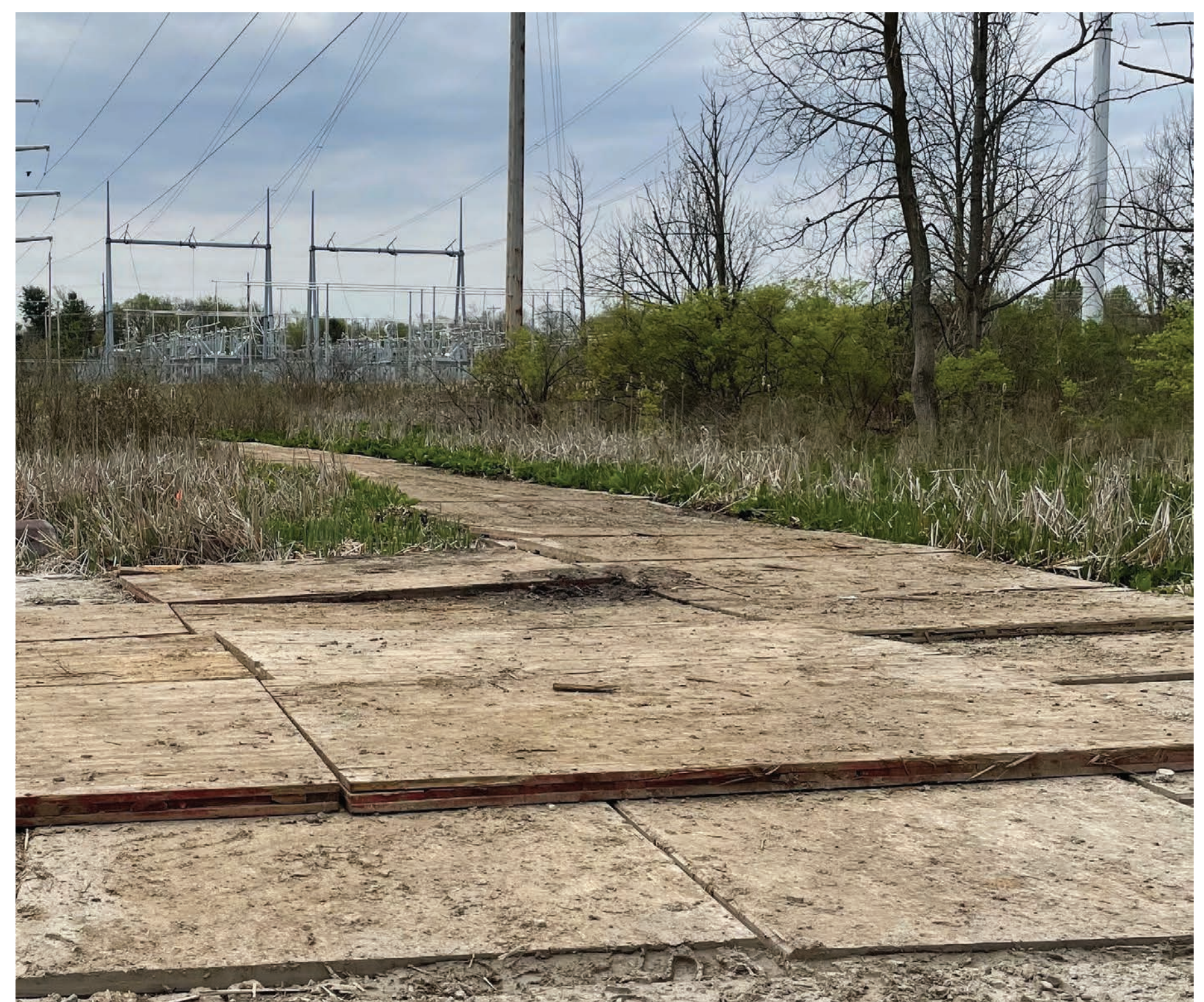
Construction mats minimize erosion of soil during construction and restoration of work areas.
